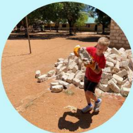
Michael (3A) helping with the construction of a kitchen oven for a local school in Kenya.
